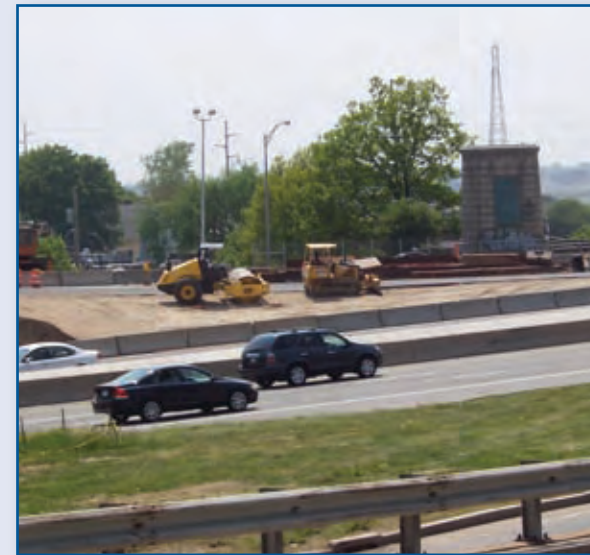
Final design for new ramps to and from Interstate 195 in the vicinity of Taunton Avenue and Warren Avenue was underway in 2007.
