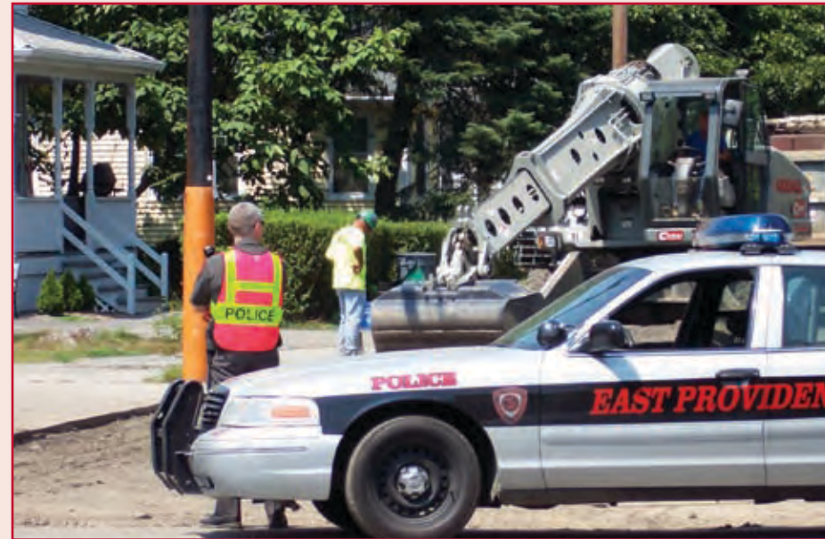
Police officers work closely with the City's Engineering and Highway Departments to provide traffic control for street and sidewalk repair projects.
